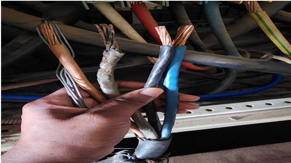
Image 2: 4 core 25mm 2 which was removed, it was supplying power from Power house to general cabinet
